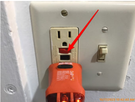
Reset button damaged
