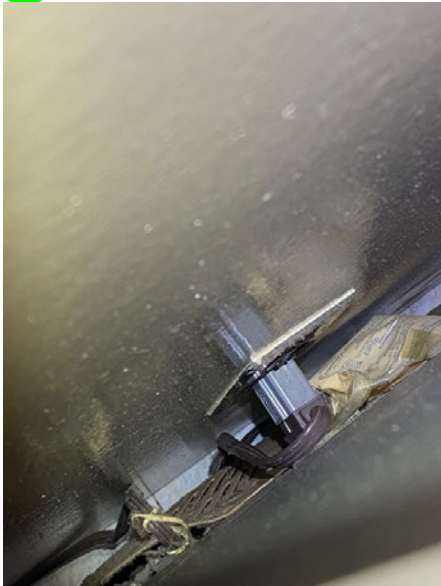
Ungrounded outlet for fridge
