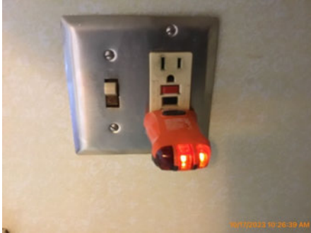
Grounded GFCI to right of sink
